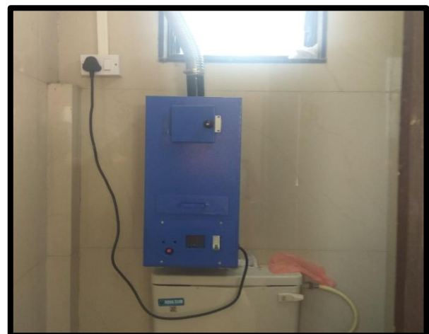
Sanitary pad incinerator
