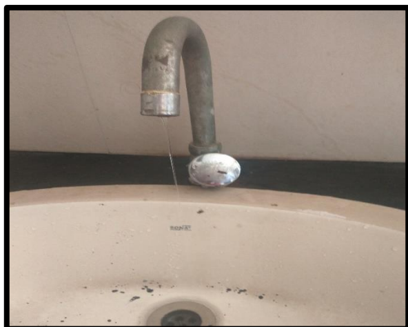
Leaking tap of wash basin
