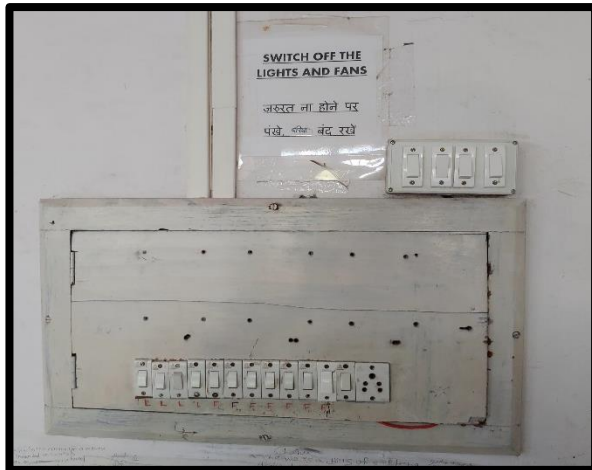
Signage above switch board
